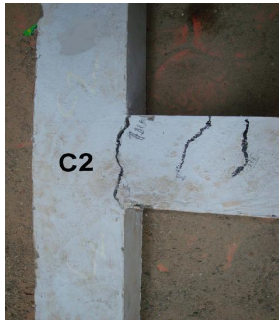
Figure 8: Crack pattern Specimens C2
