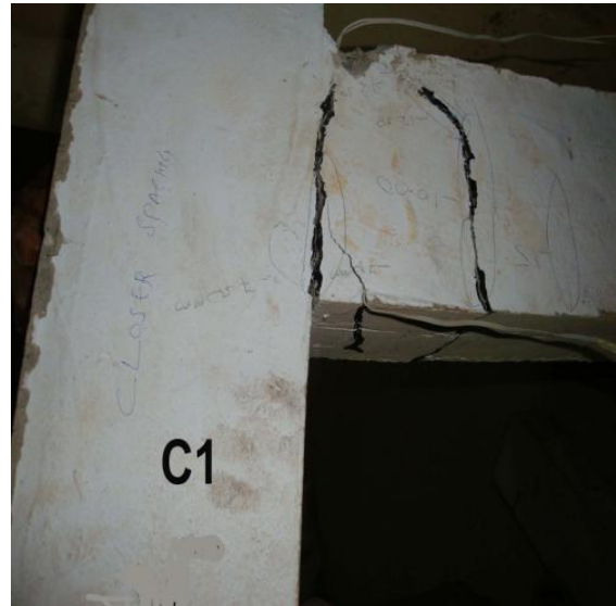
Figure 7: Crack pattern Specimens C1
