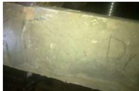
(c) Shear crack
